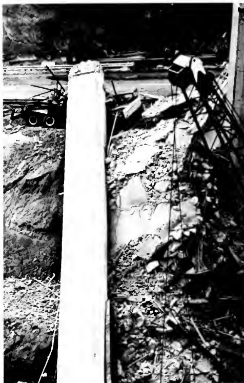
Photo 17. Collapsed span of overcrossing at the Golden State Freeway and State Highway 14 interchange [7].
